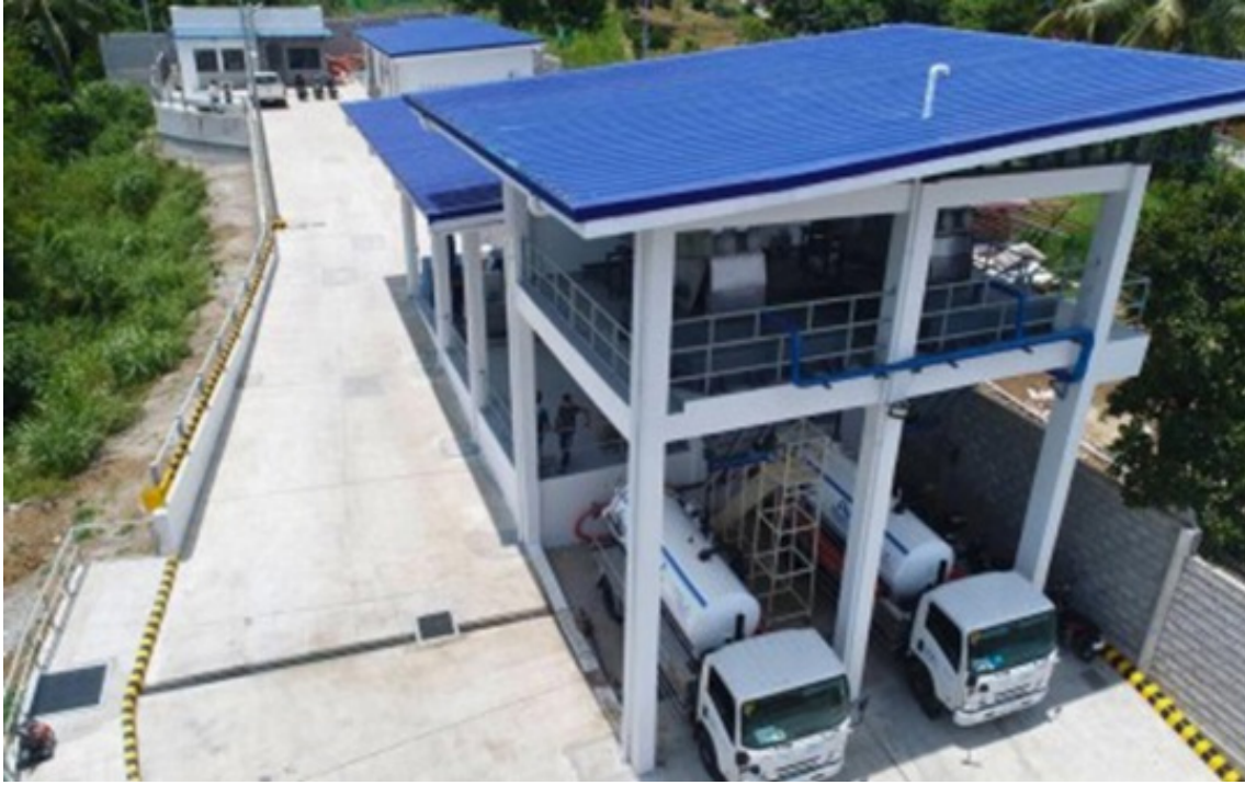
Tagaytay's first septage treatment plant (Contributed photo)
